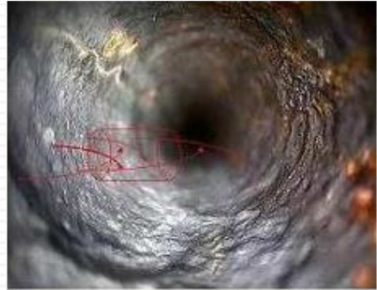
Black pipe corrosion creates air turbulence, i.e. pressure drop
